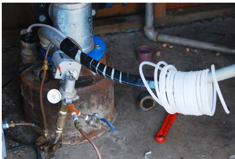
Figure 9. Polyethylene tubing deployed down well to the 213 foot level.
